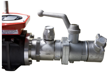
Fig. 7.1 Ball Valve to facilitate static pressure measurements
