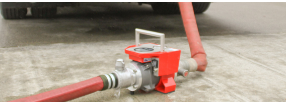
Fig. 1.4 Testing a fire pump
