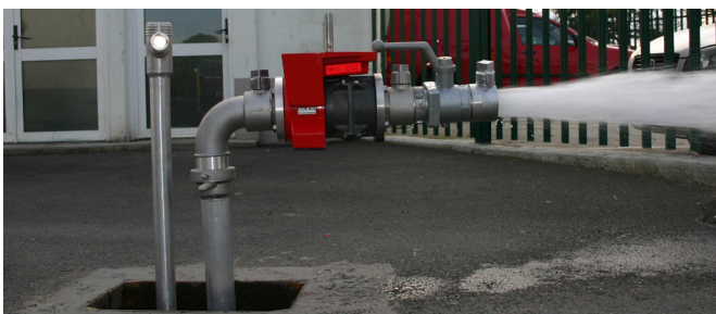
Fig. 4.3 Flow testing with ball valve to facilitate static and residual pressure measurements at Portlaoise Hospital. Photograph courtesy of Portlaoise Hospital Service
