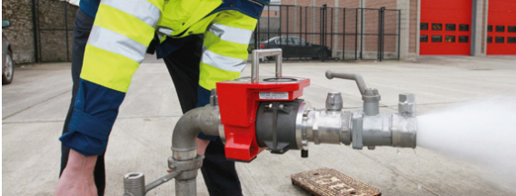
Fig. 1.2 Testing an underground fire hydrant
