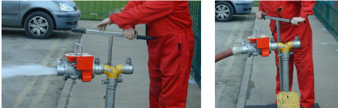
Fig. 4.1 Testing an underground hydrant using a standpipe. Photographs courtesy of Essex County Fire and Rescue Service.
